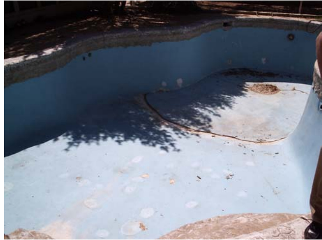
Several hollow spots are needed to be repaired
