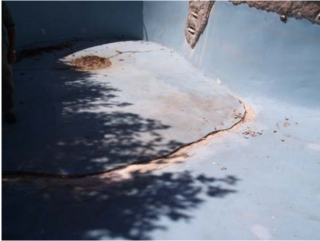
Large separation from poured concrete shown
