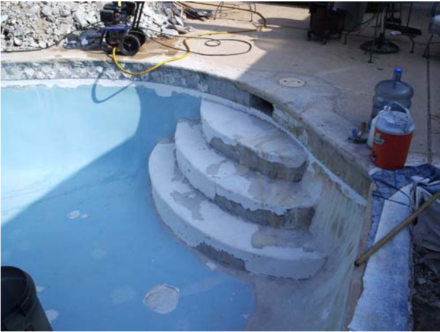
Steps were in need of repair, refurbishing
