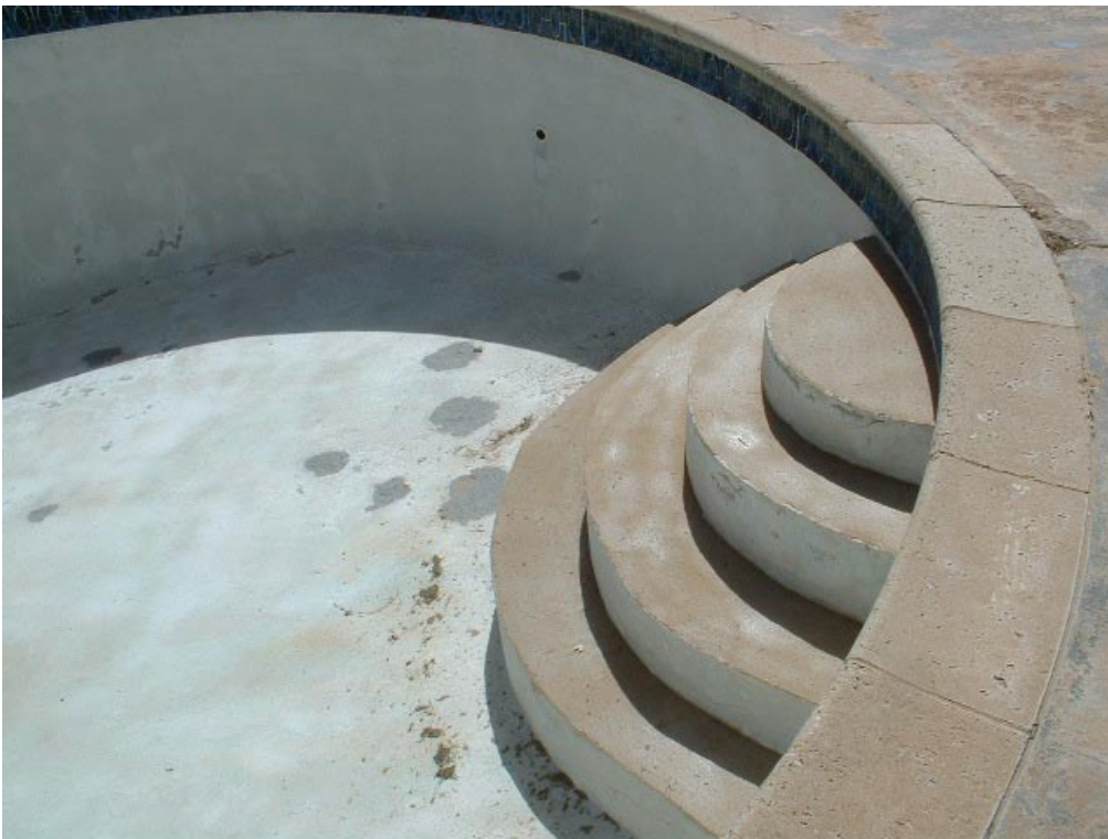
Ponderosa Apartments Pool #2: Total resurface and repair of steps using CeRam-Floor primer and silica sand at a 7:1 ratio of sand to resin
