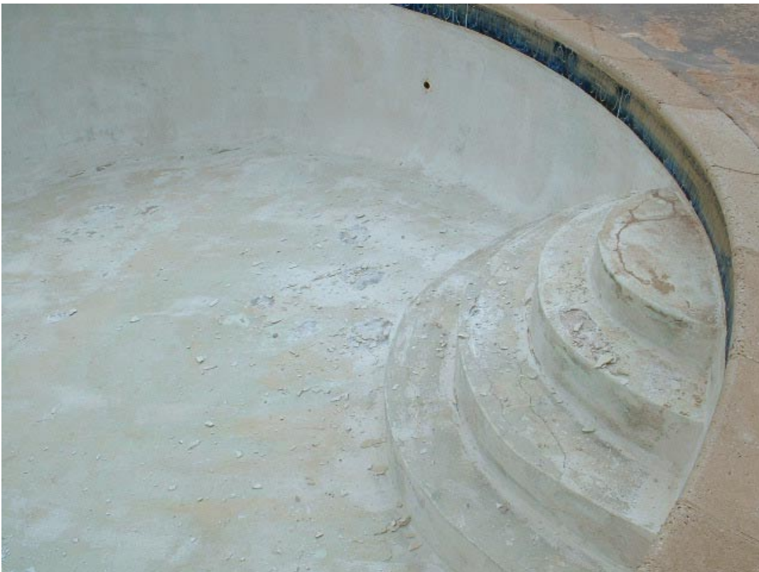
Ponderosa Apartments Pool #2: Steps in very bad condition. Cracking, spalling, etc.
