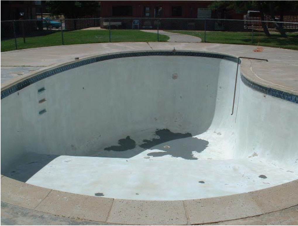
Ponderosa apartments Pool #2: Preparation via sandblasting and acid etching. Repair work performed using CeRam-Floor primer with high percentage of sand (we only had gray sand at the time)
